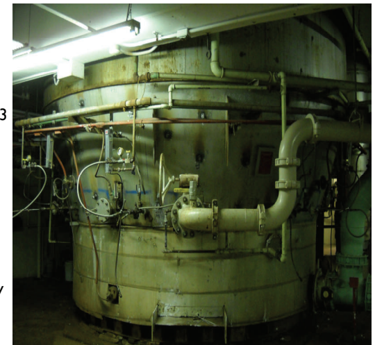
Dorr-Oliver Fluidized Bed Incinerator
